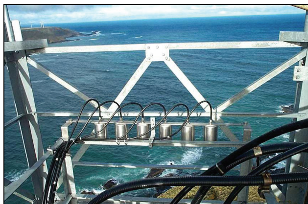
Figure 1. Image of the six new Dekabon air intake lines and rain hoods at the 75-m level on the Telstra tower.
